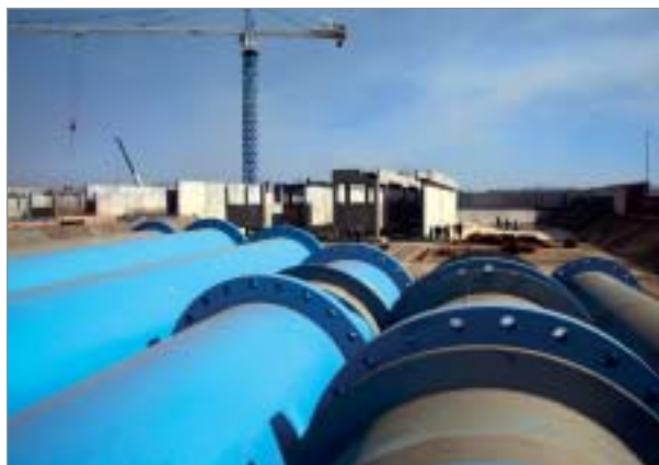
The groups' expertise with water retaining structures is evident at the Waterval waste water treatment works, south of Johannesburg
