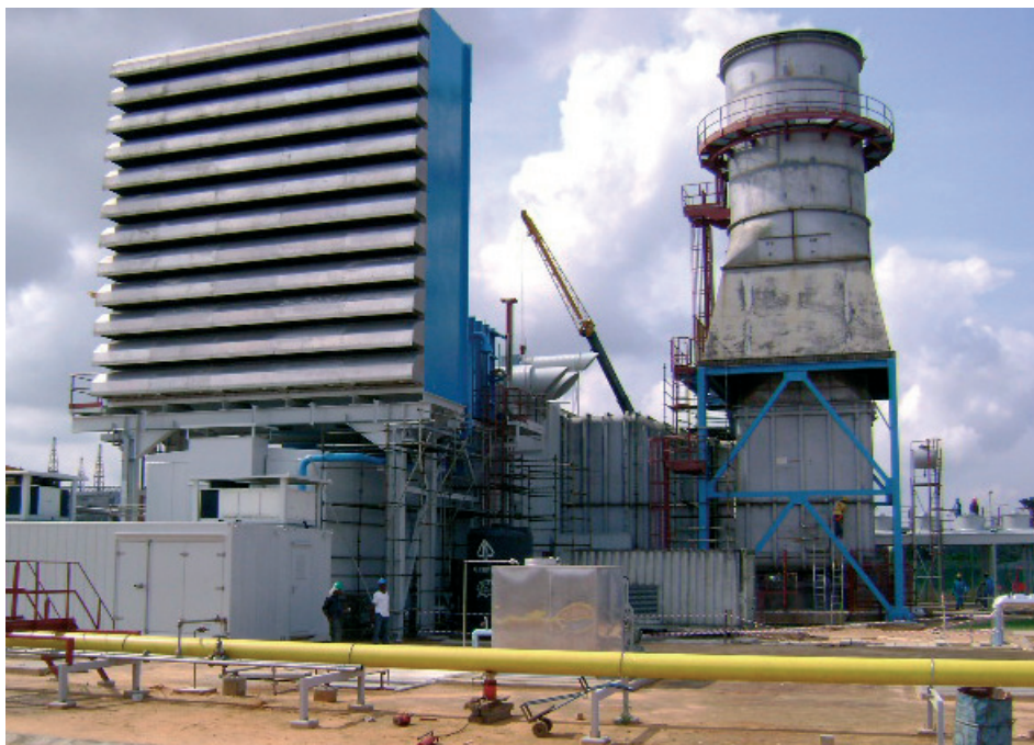
> Frame 9, Ibom gas-fired power station, Nigeria
